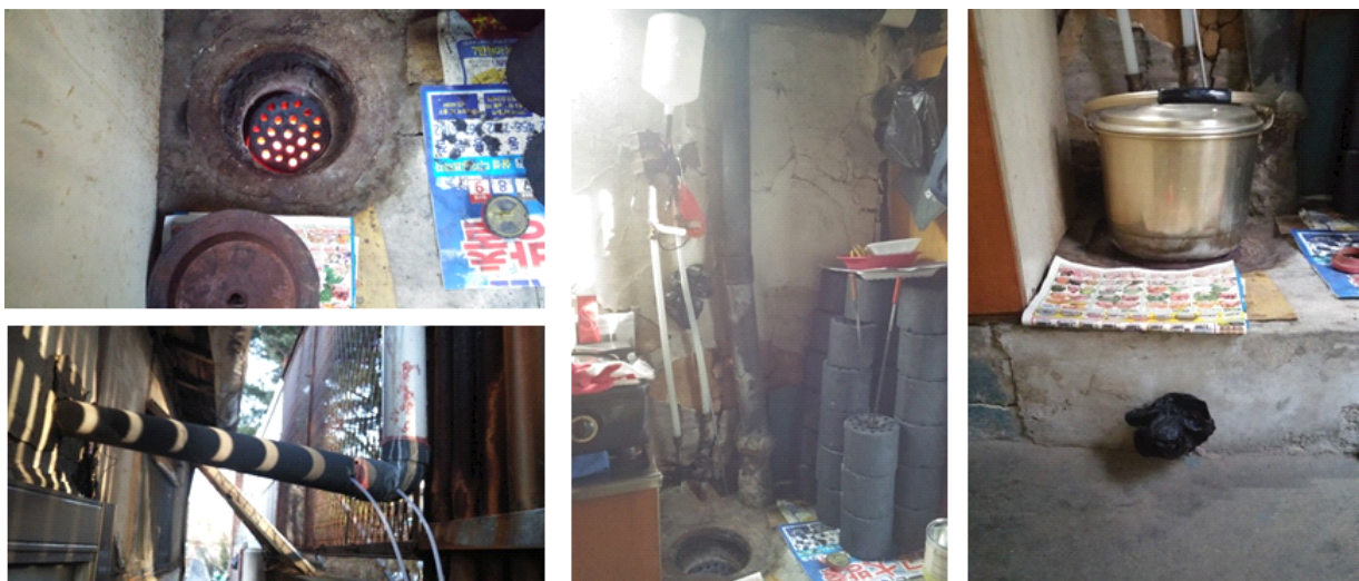
Fig. 1. Coal briquette boiler in the study site.
